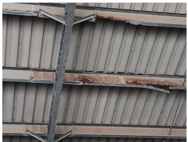
Rusted Metal Sheets & Purlins
